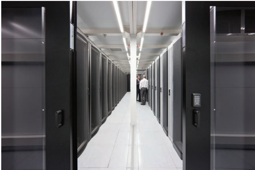
Is a data centre the responsibility of the IT manager, the network manager, or the operations director? It varies from government department to council
